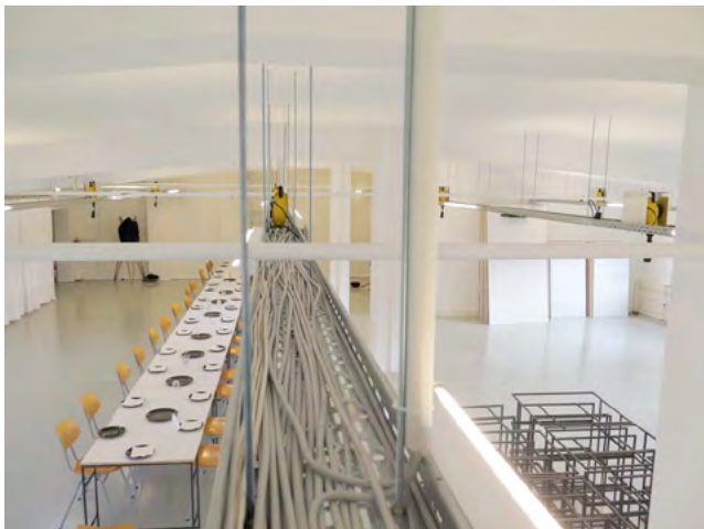
Ceiling rails provide a flexible system for electricity and light. (Photo: Fabian Scholz | Image Knowledge Gestaltung 2015)
